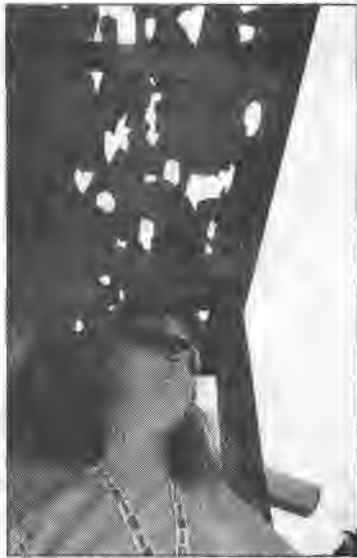
MARR BLACK/DAILY HERALD Mary Vitaioli assesses the damage after hail shot holes through the corrugated plastic roof of her deck.
