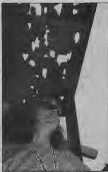
MARK BLACK/DAILY HERALD Mary Vitaioli assesses the damage after hail shot holes through the corrugated plastic roof of her deck.
